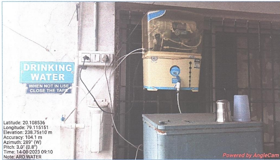
RO Water System
